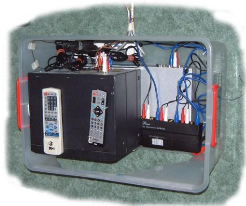
Fig 2. Fully pre-wired with all cables neatly(!) arranged, and only 5 leads leaving the package (taped together)
